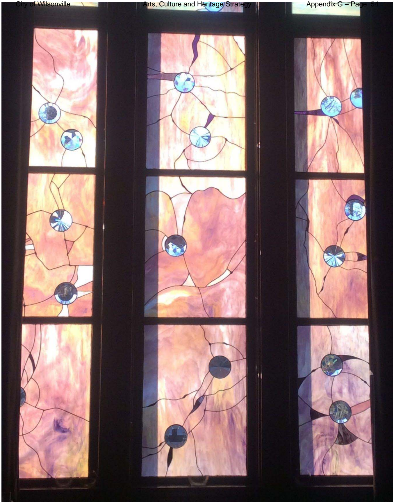
Schlicker restored the broken panes with German crystals crafted by Dan Woodward, which cast rainbows in the sunlight. Some panes were made to look broken so that all the windows match.
