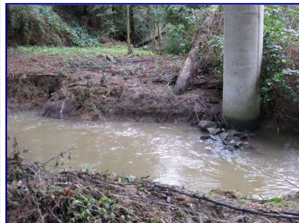
Bank erosion near Wilsonville Road piling
