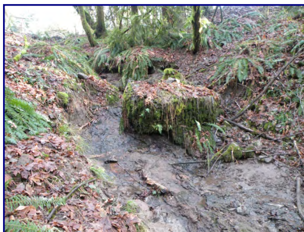
Bank erosion downstream from the Gesellschaft well
