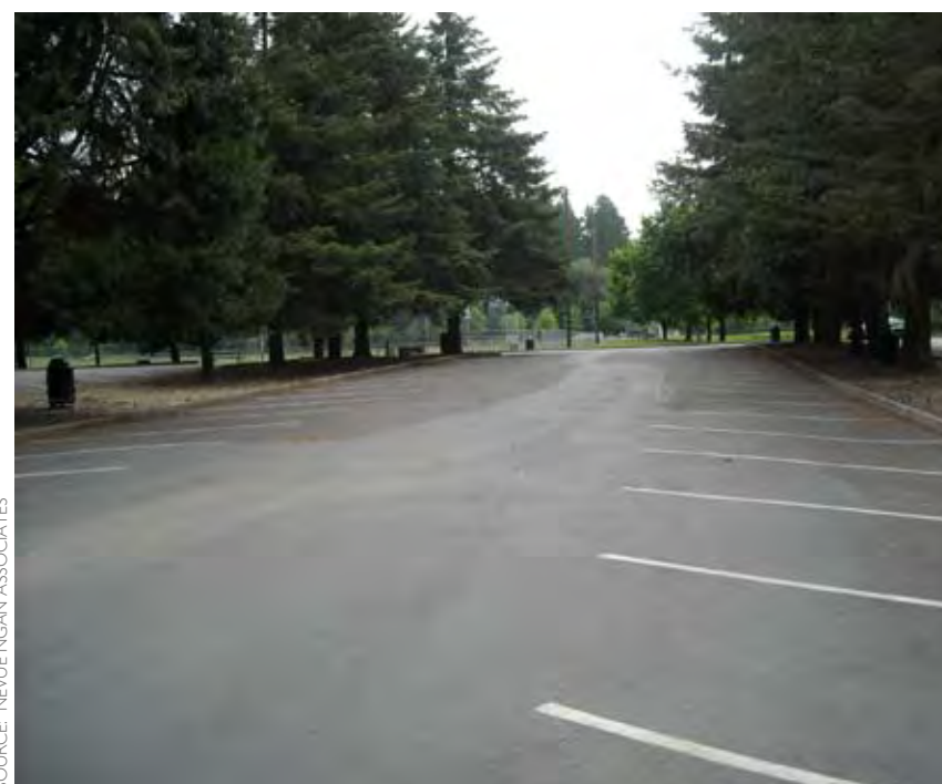
Existing Parking Lot Conditions
