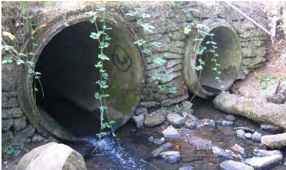
Figure #: Stormwater gains speed as it flows through pipes designed to efficiently carry it away.
