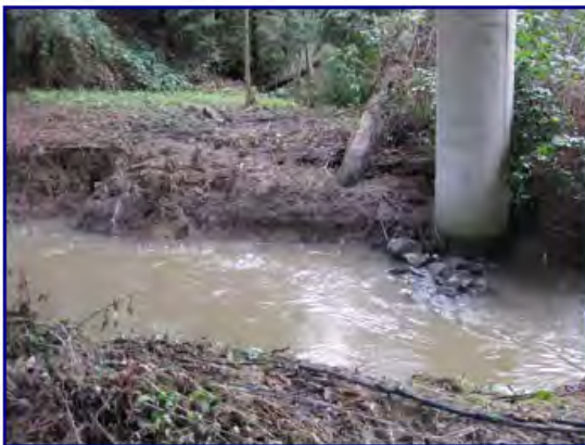
Bank erosion near Wilsonville Road piling
