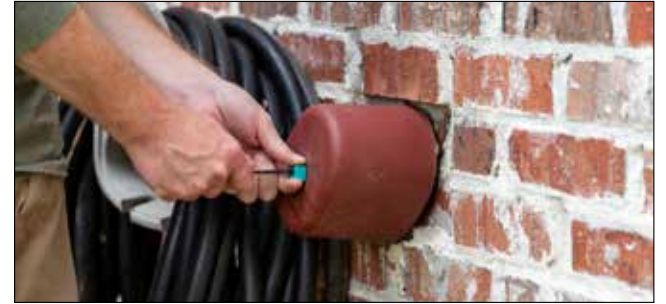
Covering exposed hose bibbs is one easy way to reduce your chance of suffering a burst water pipe.
