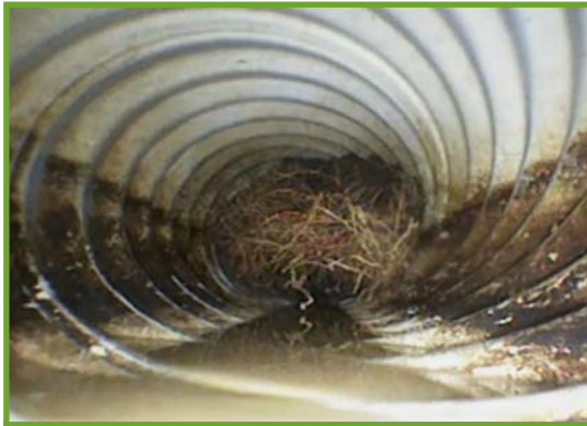
Before— roots obstructing flow
