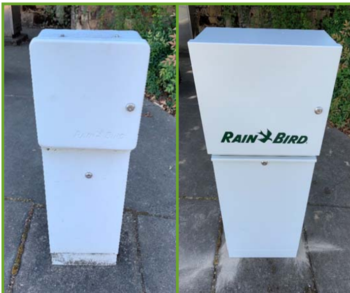
Irrigation Controller Upgrade
