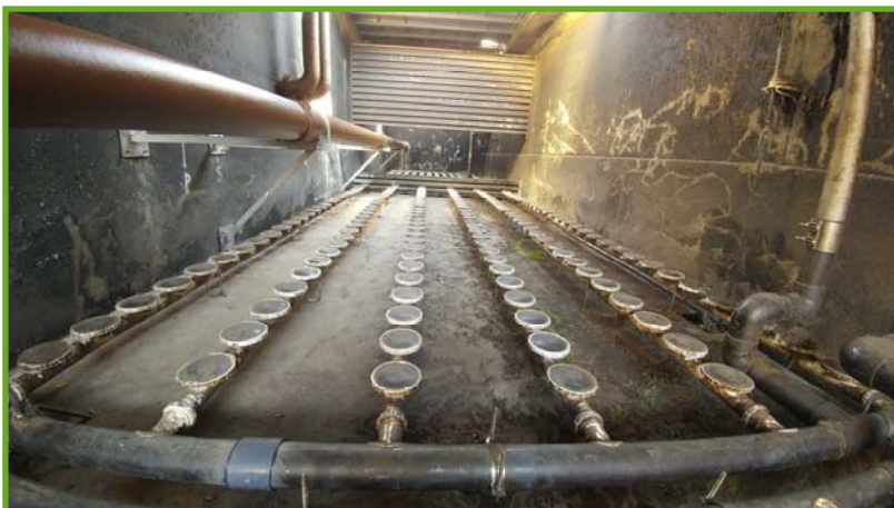
View inside of aeration basin looking from south to north—baffle wall at the far end separates the anaerobic zone (far) from the aerobic zone (near). Brown pipe on left side of basin recirculates activated sludge back to the anoxic area
