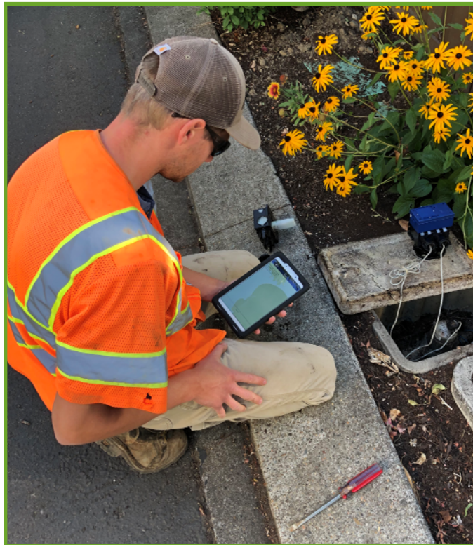
AMI radio installation
