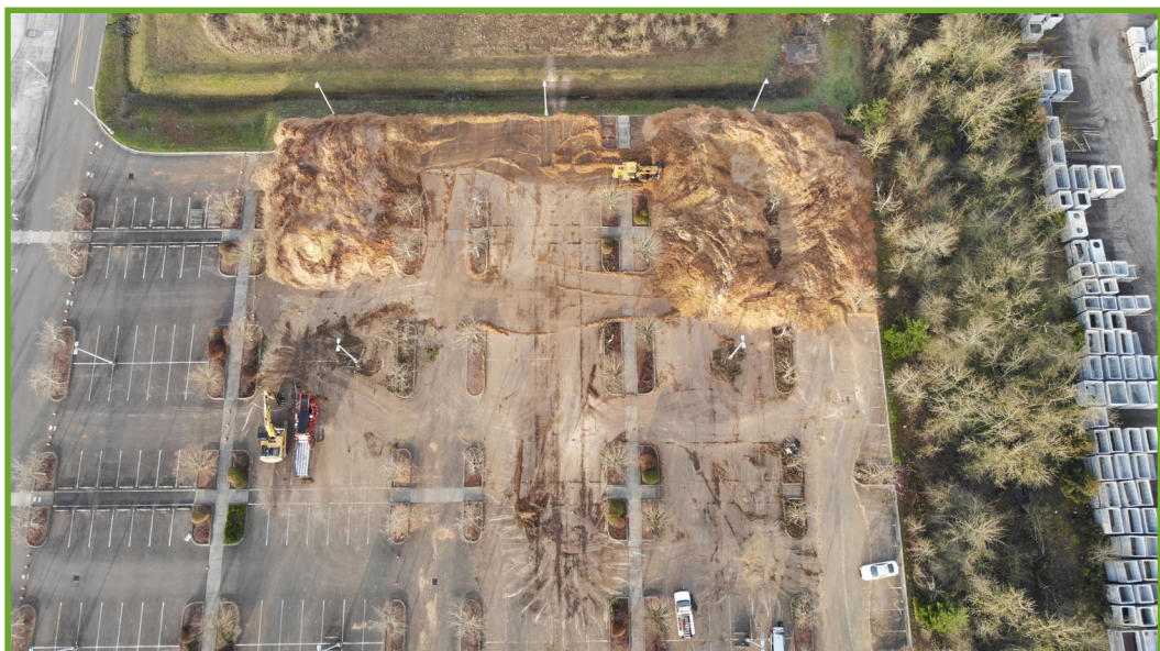
After —Chips remaining at the debris site looking to the west
