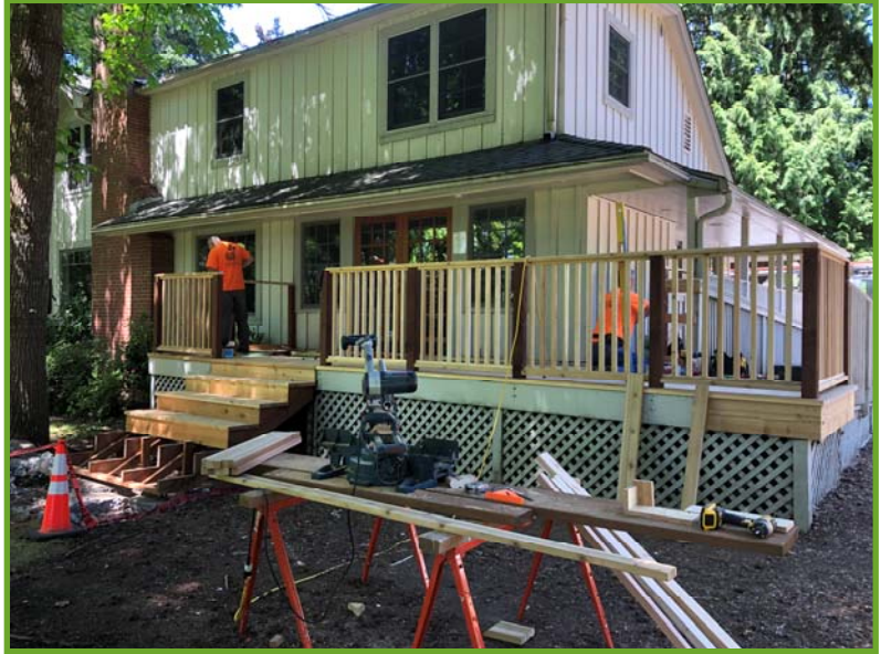
Facilities Supervisor Matt Baker and Technician Javid Yamin, put the final rail pickets in place
