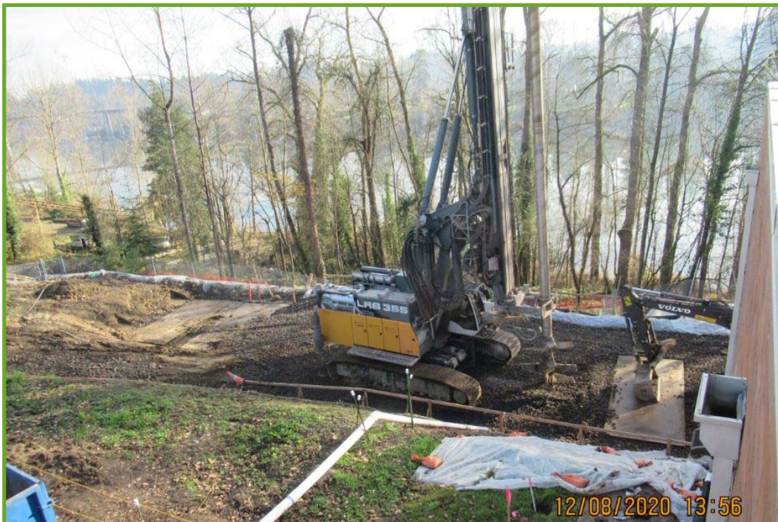
Drill rig for deep soil mixing which will provide seismic stability of the Willamette River bank.
