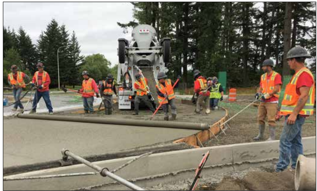
Workers pour, roll flat and smooth out concrete road surface for enlarged roundabout at the intersection of Kinsman and Boeckman Roads.
