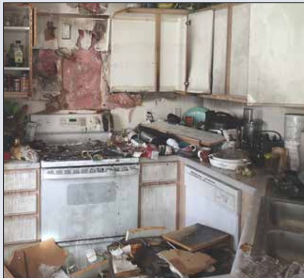
This kitchen fire was caused by unattended cooking at a home in Wilsonville this April.
