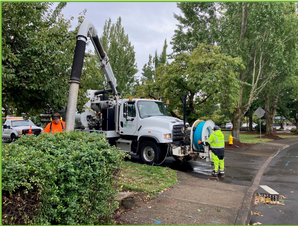
Using the vector truck to assist the Water team with repair work
