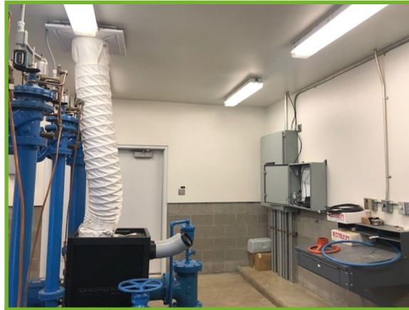
Portable A/C unit at work
