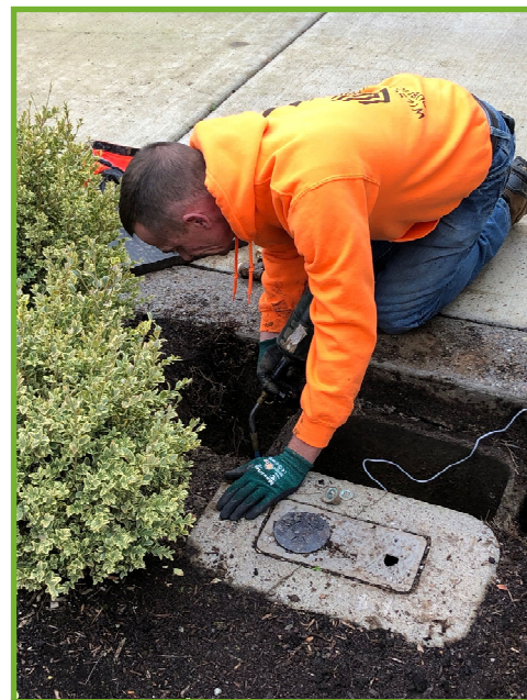
Checking a residential meter
