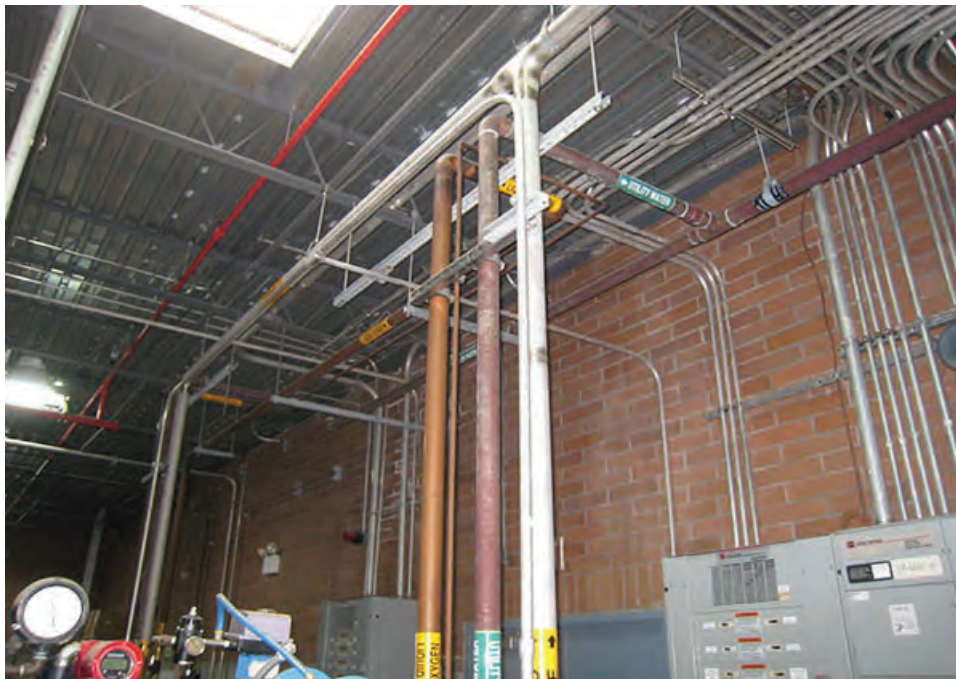
Photo 38 – S14 – The ozone and LOX piping at the Ozone Generation Room lacks seismic bracing.
