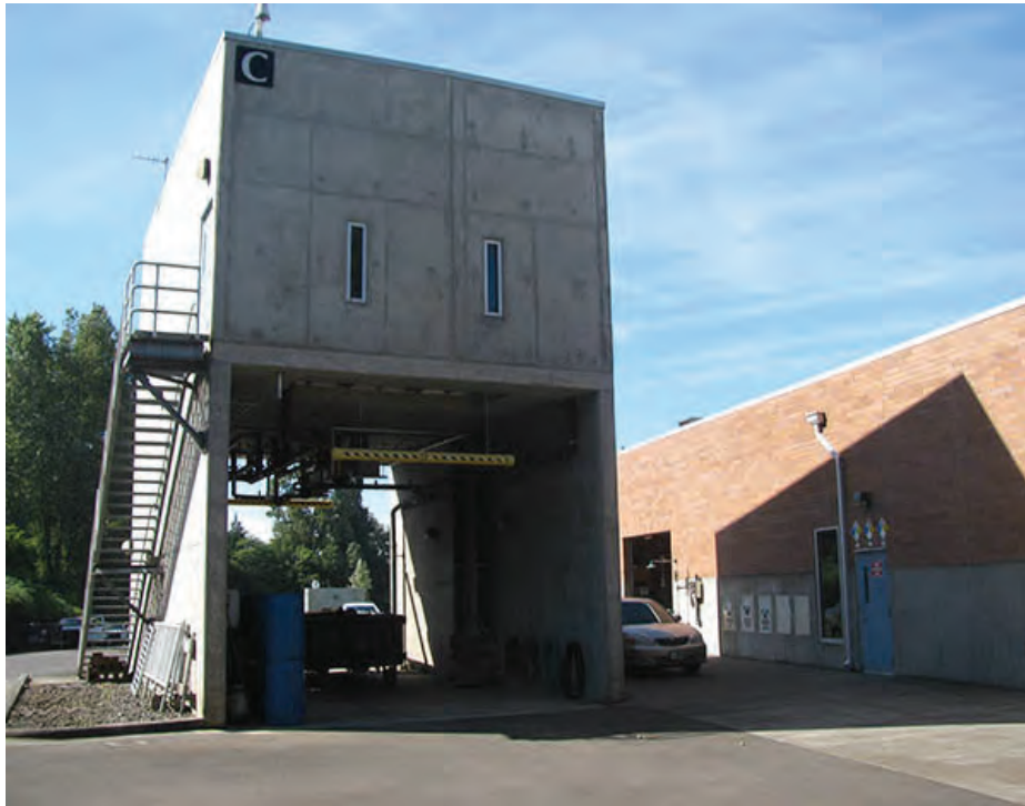
Photo 31 – S7 – The Solids Dewatering Building has no lateral load resisting system at the lower level in the east-west direction.
