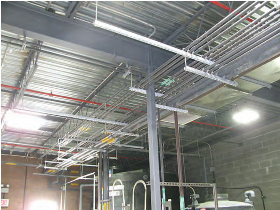
Photo 12 – LS6 – Chemical piping passing directly over the egress route to the east door at the Chemical Storage Room.
