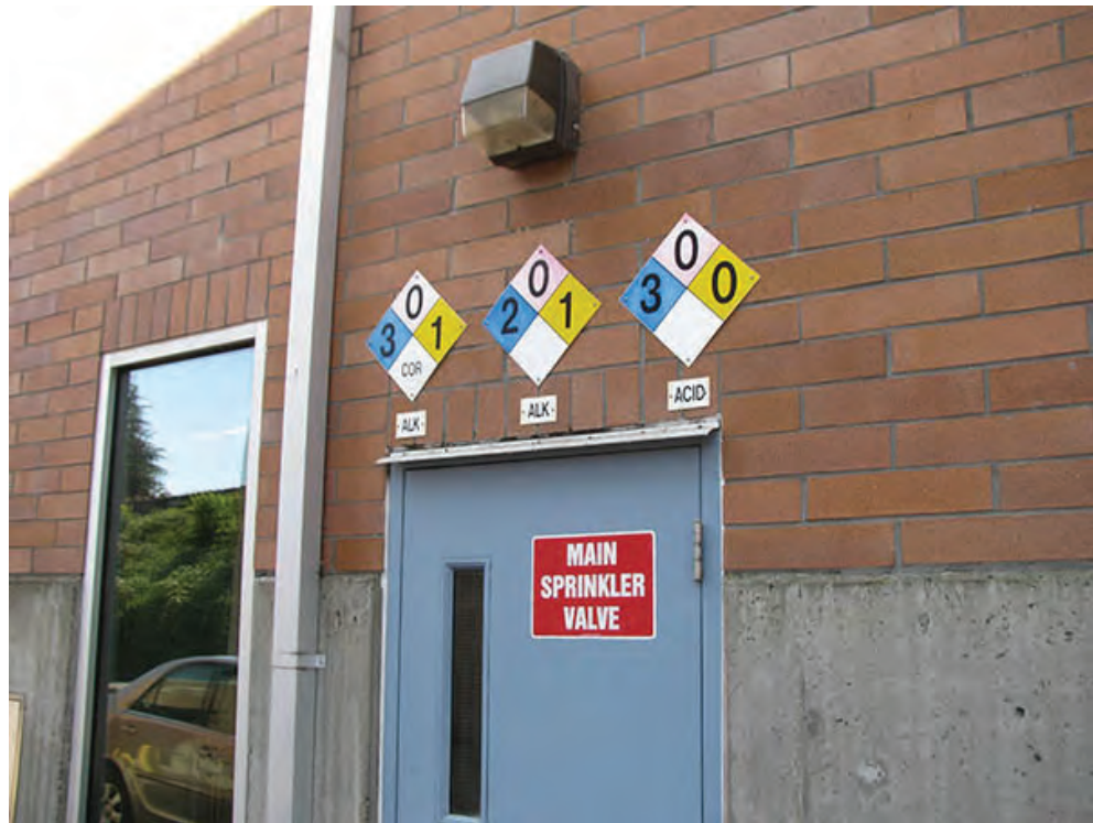
Photo 4 – LS2 – Color coded safety warning signs are faded at the east wall of the Chemical Storage Room.
