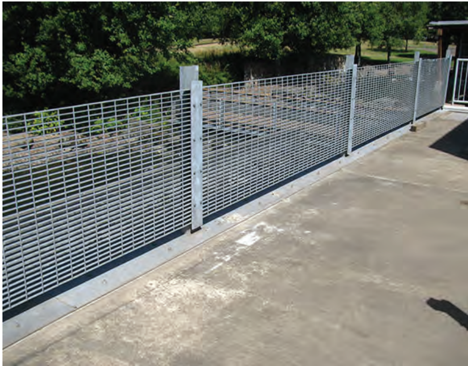
Photo 15 – LS8 – West guardrail on top of the Actiflo™ Basin lacks a kick plate and it is located over a public walkway.
