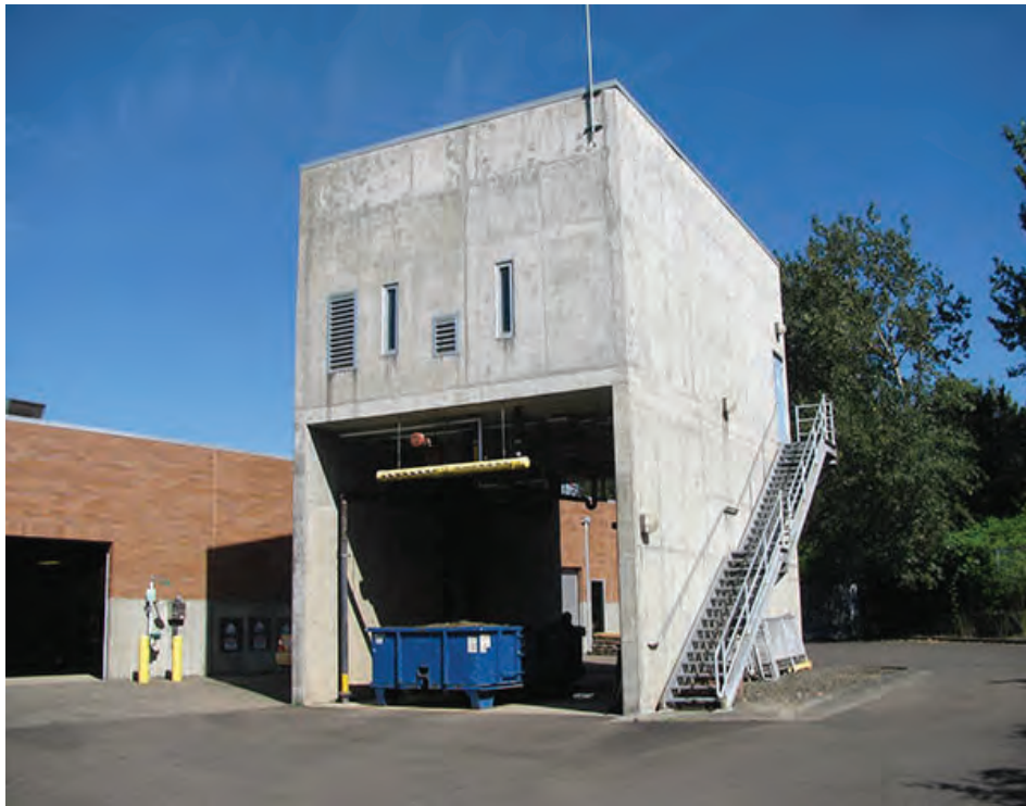
Photo 25 – LS14 – The Solids Dewatering Building does not have any overflow scuppers visible.
