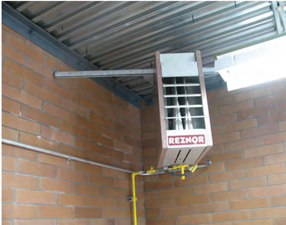
Photo 33 – S10 – The space heater at the Washwater Pump Station is suspended and unbraced for seismic loads.
