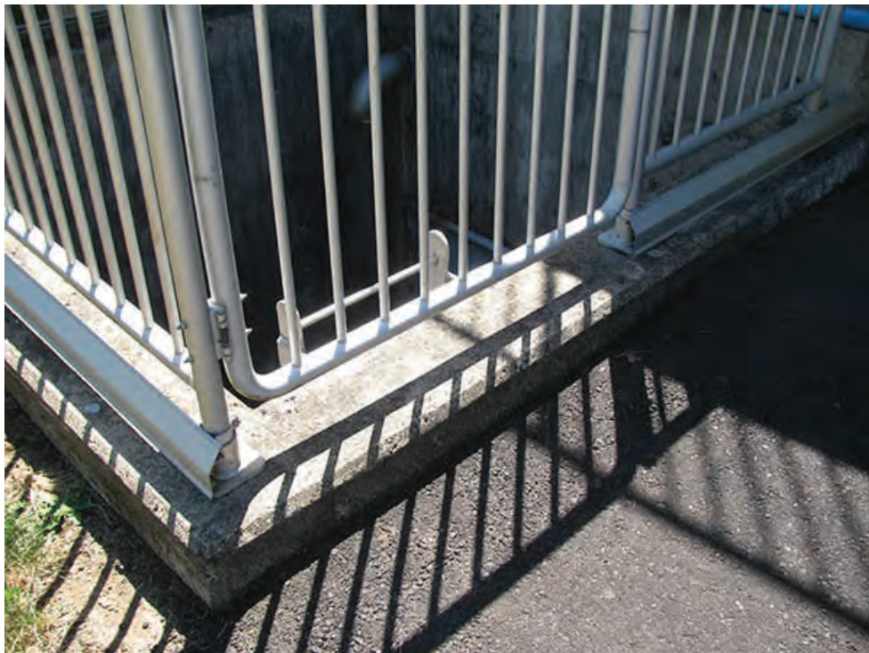
Photo 16 – LS8 – Gate at the Filter ladder pit lacks a kick plate.
