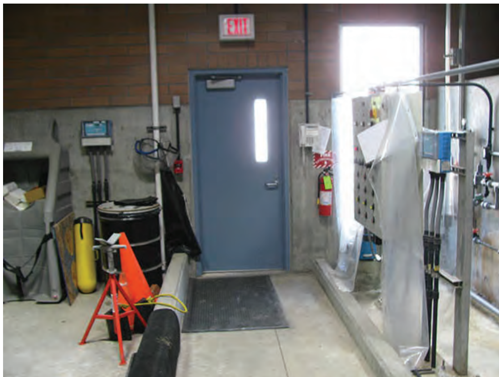
Photo 10 – LS5 – Group occupancy H at the Chemical Storage Room requires panic hardware on the exit doors (the east door shown).
