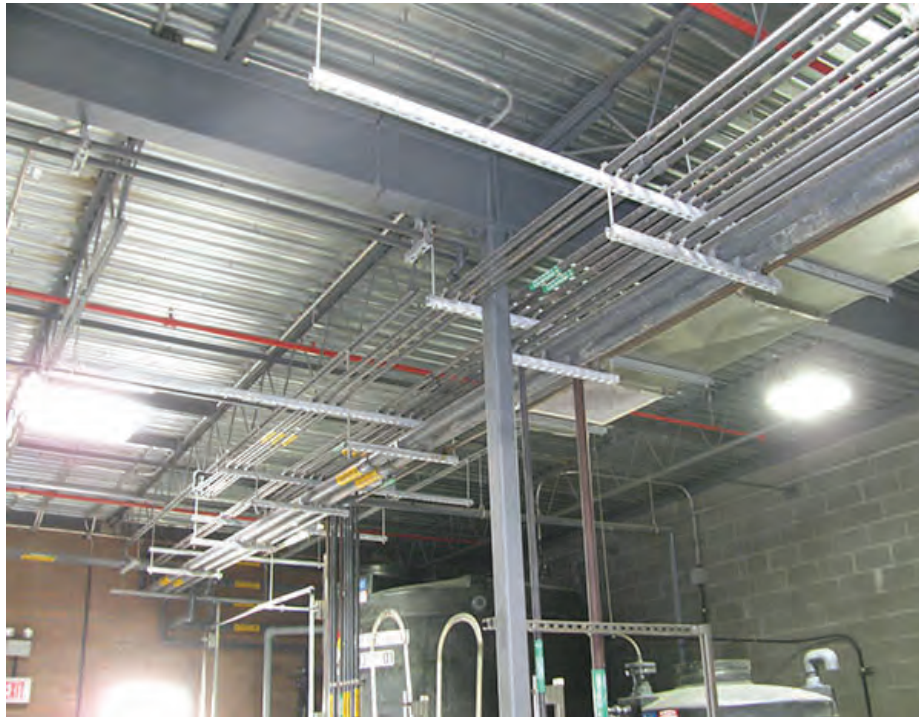
Photo 37 – S13 – The chemical piping at the Chemical Storage Room lacks transverse seismic bracing.
