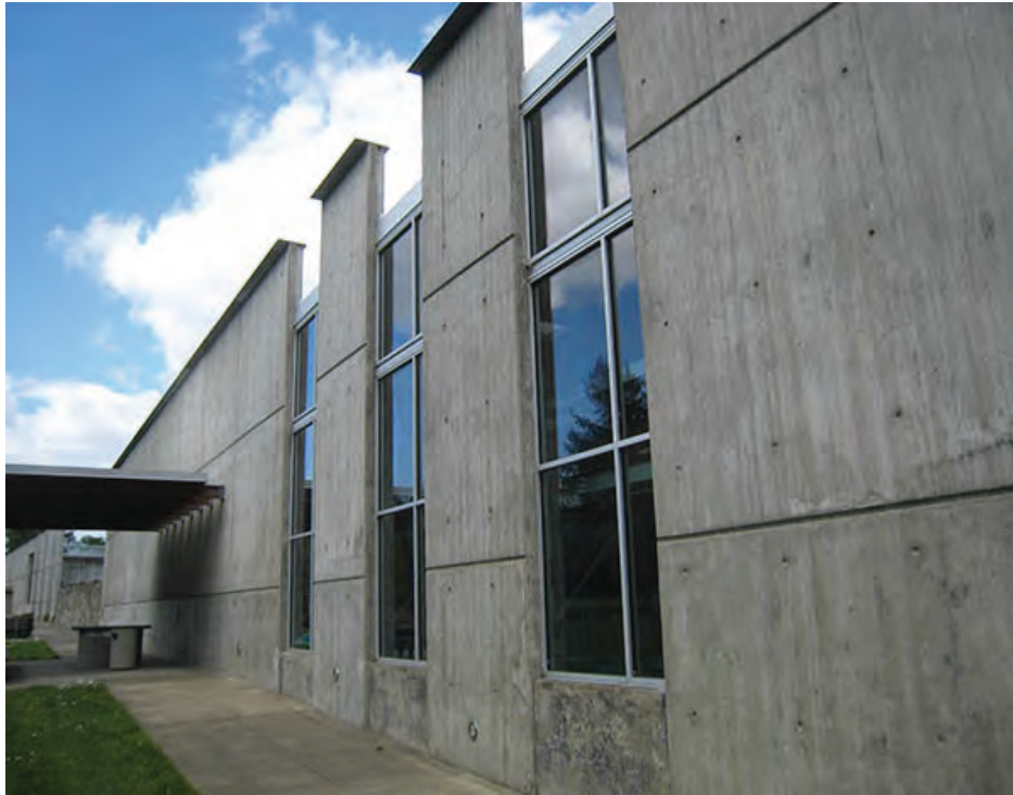
Photo 29 – S5 – Diaphragm chord splices at the windows along the west wall require strengthening.
