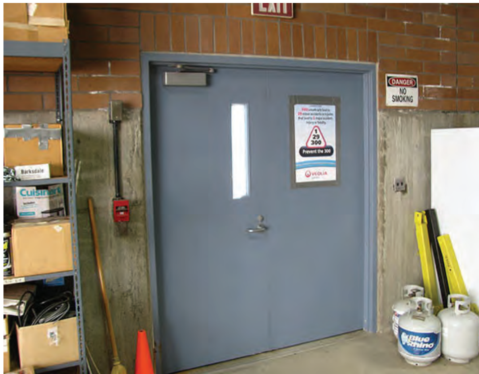
Photo 9 – LS5 – Group occupancy H at the Ozone Generation Room requires panic hardware on the exit doors (one of the south doors shown).
