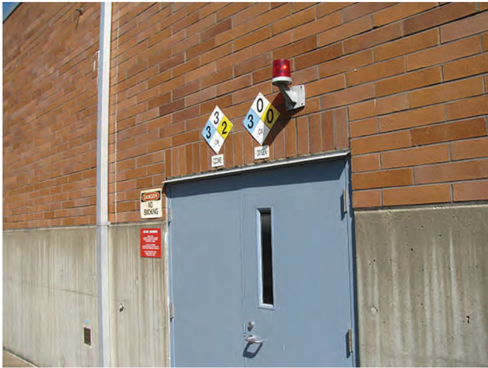
Photo 3 – LS2 – Color coded safety warning signs are faded at the south wall of the Ozone Generation Room.
