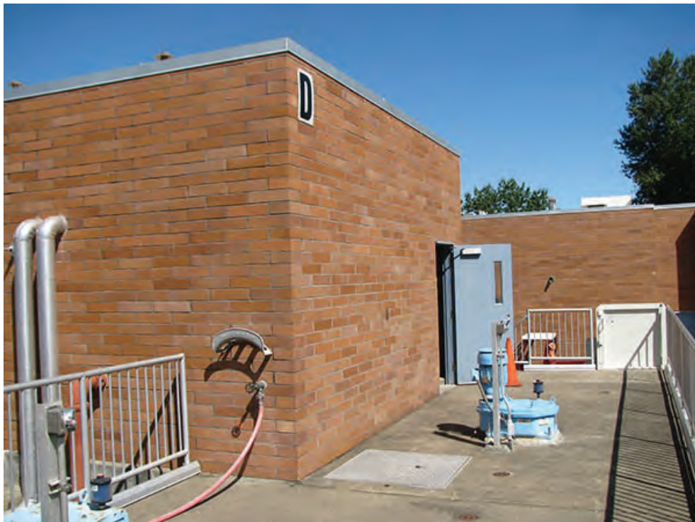
Photo 14 – LS7 – Door at the Actiflo™ Room was found propped open.
