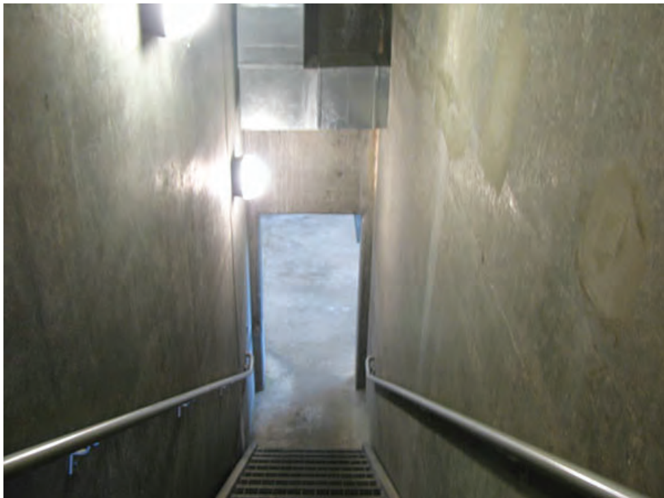
Photo 22 – LS12 – Entrance to the Filter Gallery. The door is located at the top of the stairs.
