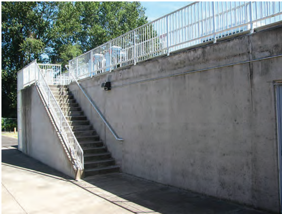
Photo 6 – LS3 – Guardrail at the north Filter staircase is less than 42 inches in height.
