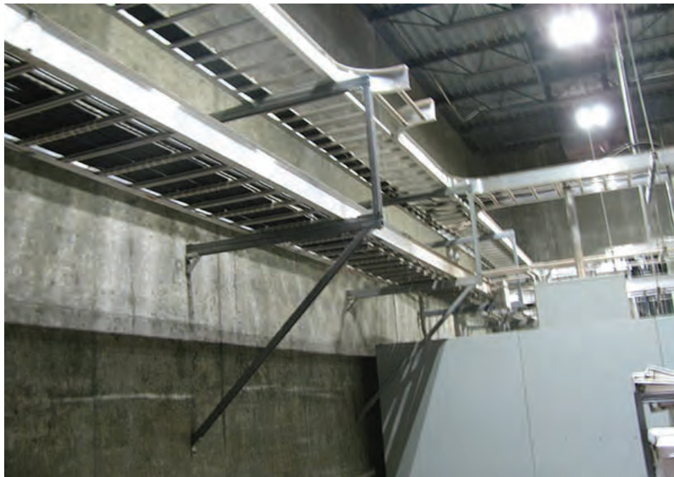
Photo 36 – S12 – The cable tray within the High Service PS lacks longitudinal seismic bracing.
