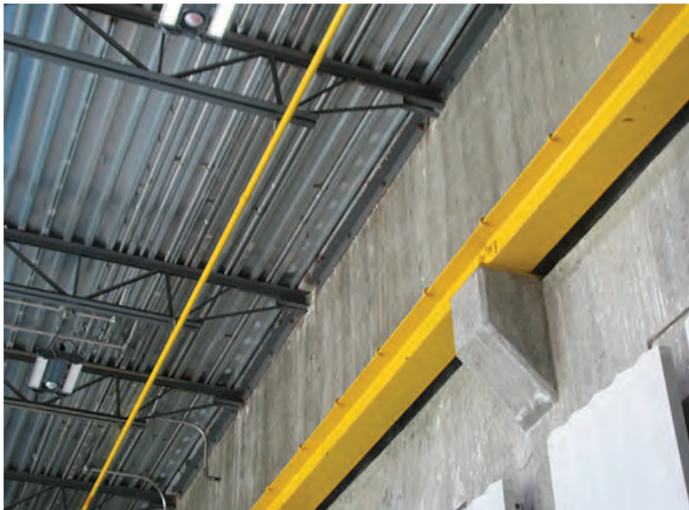
Photo 28 – S3 – The roof joist wall anchorage to the walls at the High Service Pump Station lack capacity to meet seismic performance goals.
