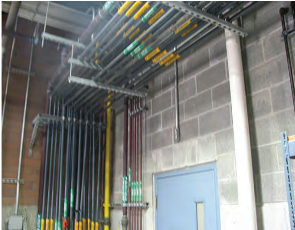
Photo 11 – LS6 – Chemical piping passing directly over the west door at the Ozone Generation Room.
