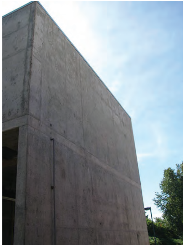
Photo 26 – LS14 – The Solids Dewatering Building does not have any overflow scuppers visible.
