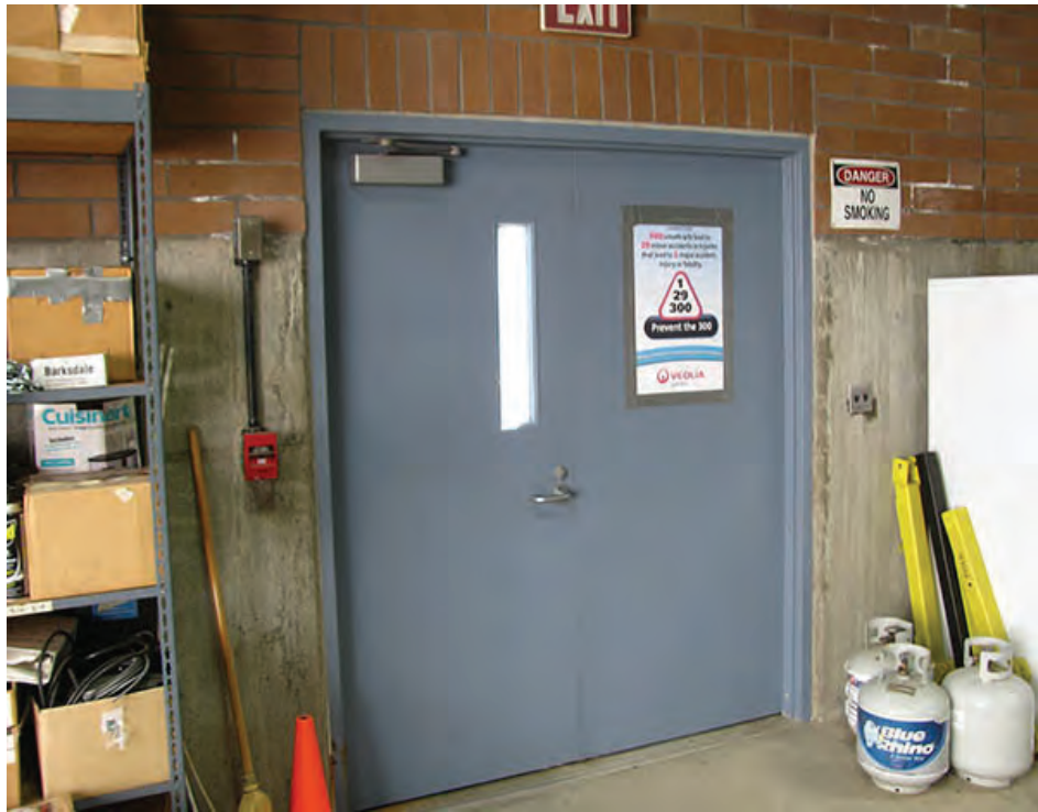
Photo 27 – LS15 – The southeast door that exits from the Ozone Generation Room does not have an emergency shut-off switch for the ozone generation equipment.
