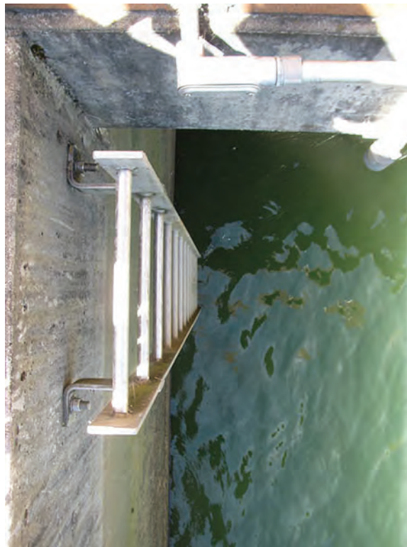
Photo 24 – LS13 – The access ladder to the Waste Washwater EQ Basin does not have any tie-offs for a fall restraint system.
