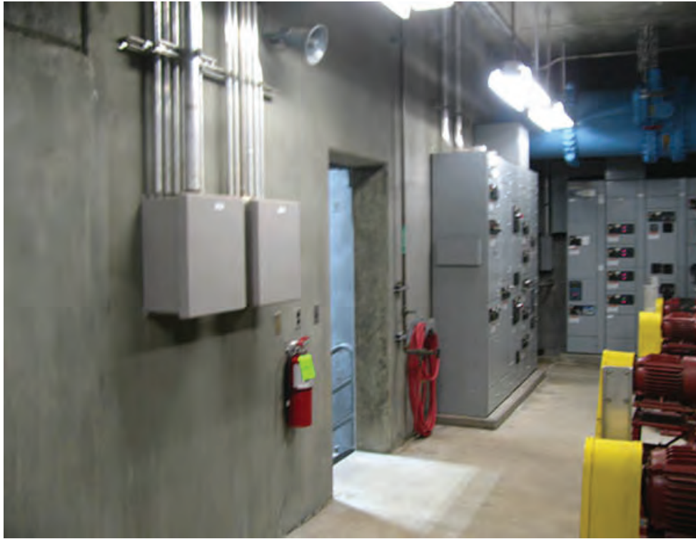
Photo 7 – LS4 – The Actiflo™ gallery has electrical service rated at 1200 amps or higher requiring panic hardware on doors.
