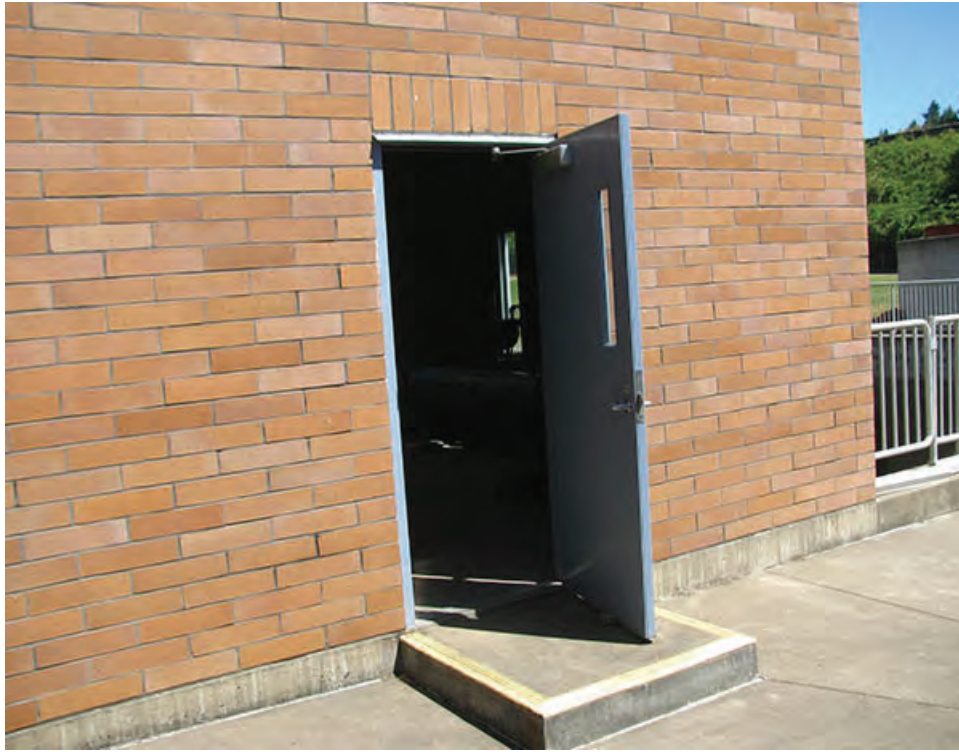
Photo 13 – LS7 – Door at the Waste Washwater Pump Station was found propped open.
