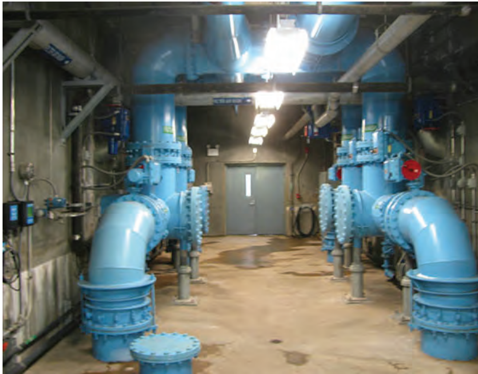
Photo 23 – LS12 – The east end of the Filter Gallery has a double door that leads out to a ladder pit.
