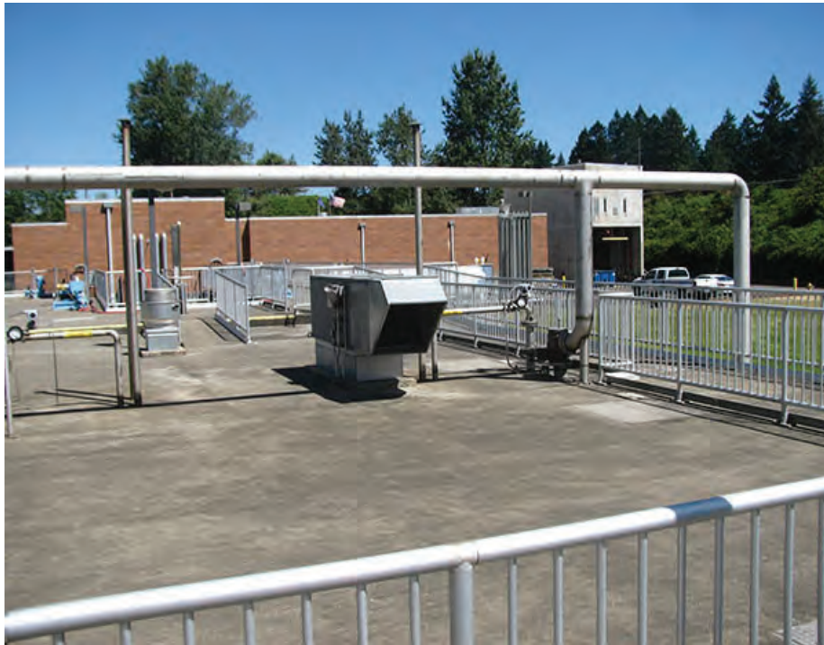
Photo 35 – S11 – The ozone destruct piping lacks seismic bracing at the top of the Ozonation Basin.
