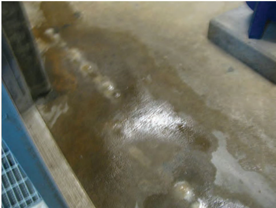
Photo 18 – LS9 – Water on the floor of the south blower room at the Filter Gallery due to active leaks from the water channels above.
