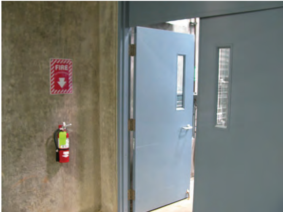
Photo 8 – LS4 – The Switchgear Room at the High Service Pump Station has electrical service rated at 1200 amps or higher requiring panic hardware on doors
