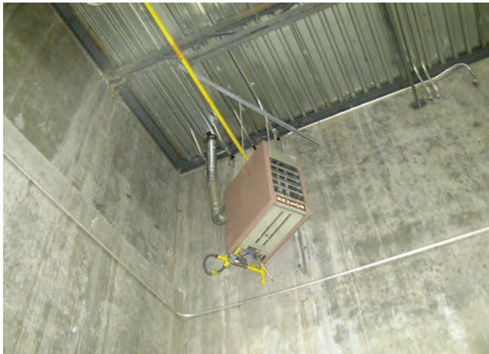
Photo 34 – S10 – The space heater at the Switchgear Room at the High Service PS is suspended without any seismic bracing.
