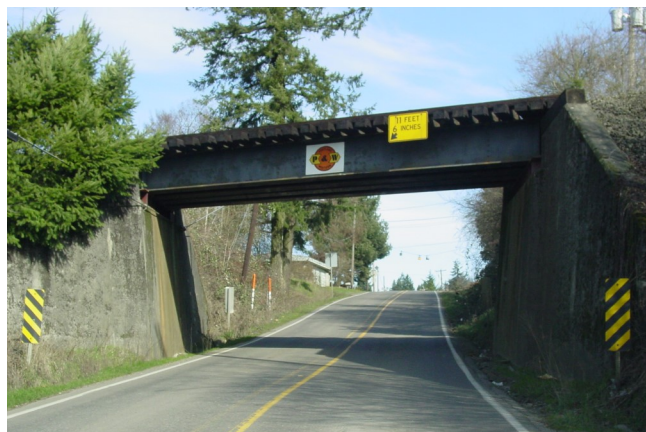
The railroad bridge over Grahams Ferry Road has limited horizontal and vertical clearance. This creates a safety hazard, particularly for bicyclists, pedestrians, and freight traffic.
