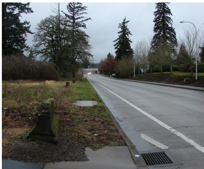
Freeman Drive between 95th Avenue and businesses lacks sidewalks on the south side.
