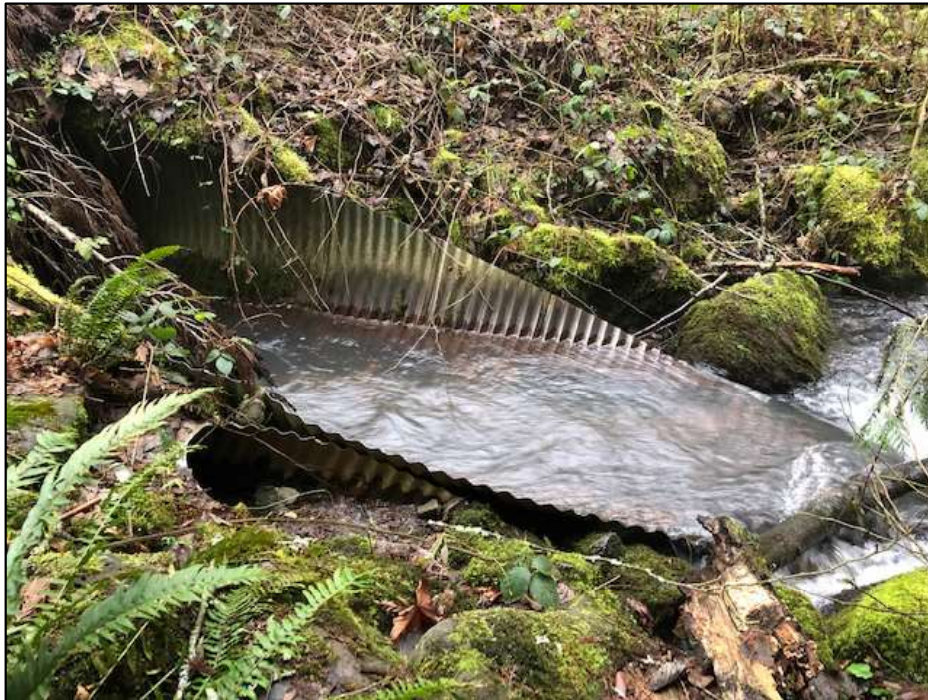
Main Large Corrugated Metal Pipe (CMP) Culvert conveys creek flows under the Road
