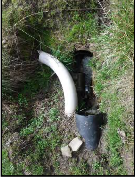
Photo F. View of 18-inch culverts at the Wetland A boundary. (Photo taken 3/29/2019)
