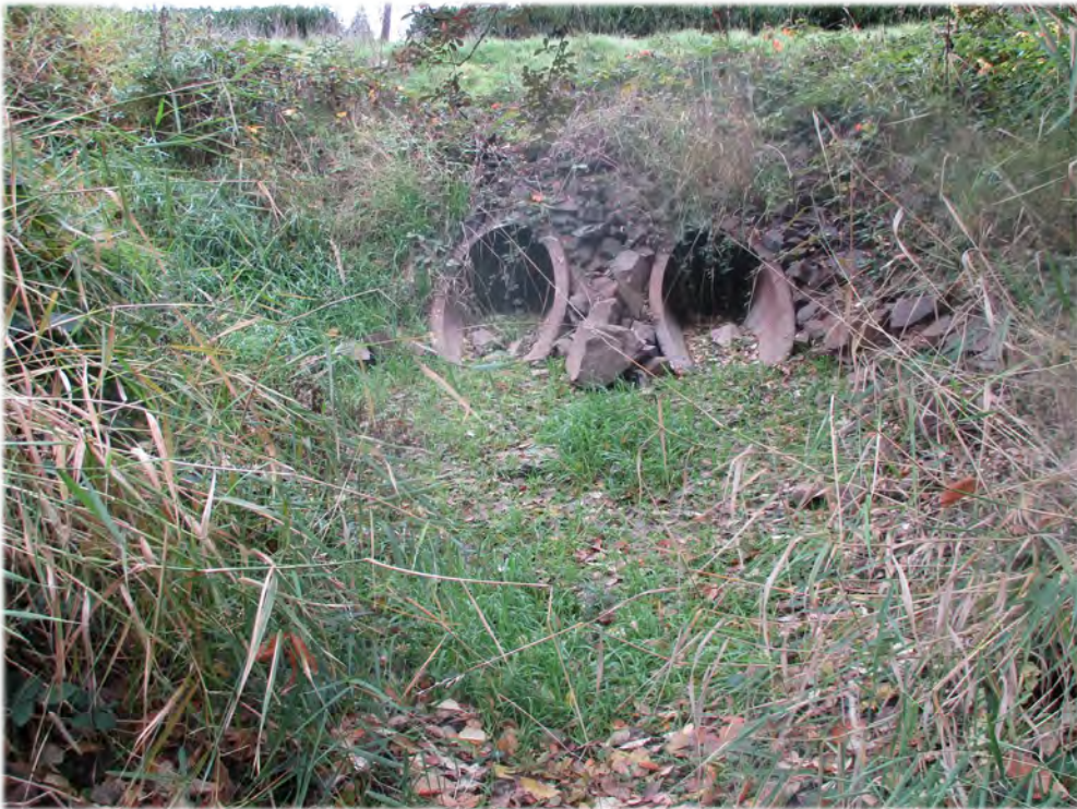
Photo Point 5. From the northern portion of Tapman Creek (wetland drainage) facing north toward double culverts (photo date: 10/23/2019).
