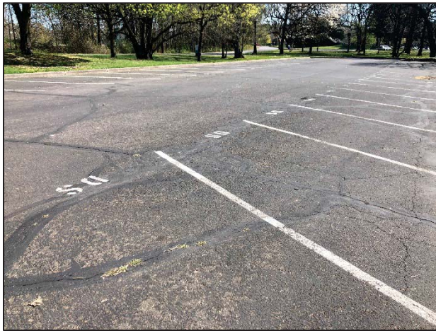
Photo 3: North Parking Bay –Random/ Transverse/ Longitudinal Cracking
