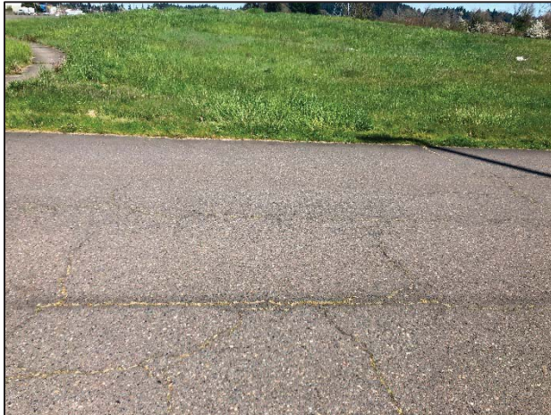
Photo 1: North Entrance Drive – Fatigue Cracking
