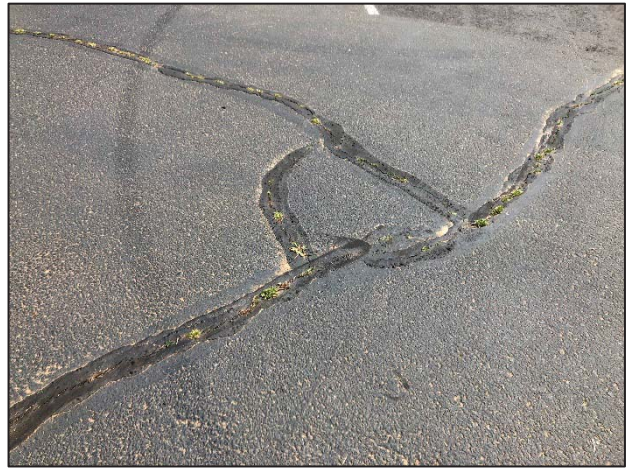
Photo 4: North Parking Bay – Crack Seal closeup
