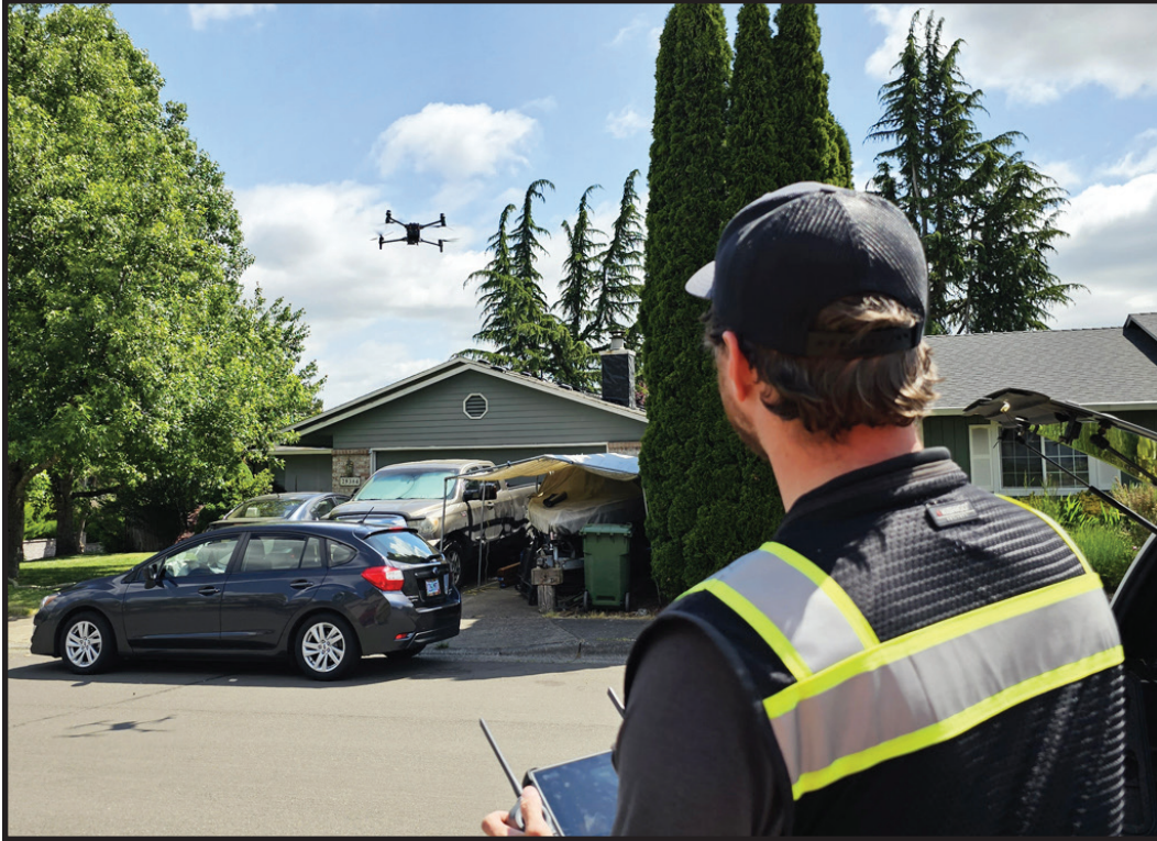
Building staff performing an inspection of new rooftop solar panels with the use of a drone.
