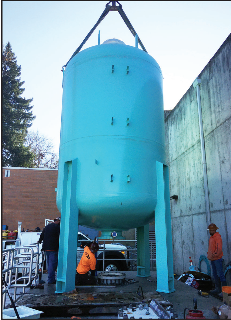
Surge tank installed at the Water Treatment Plant
