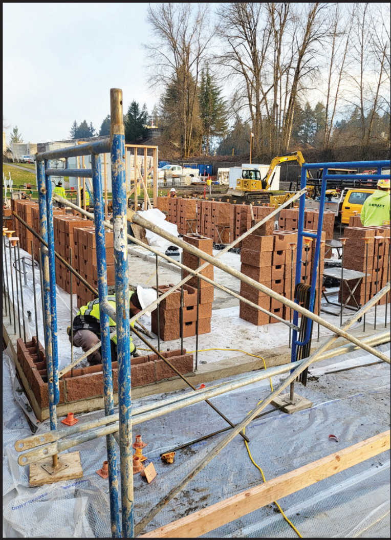
Wall construction begins on the electrical switchgear building at the Water Treatment Plant expansion (CIP #1144).
