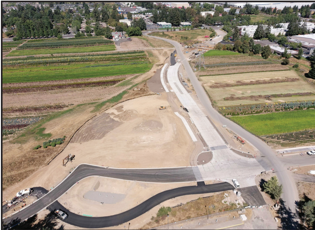
Work was staged to keep the existing roadway open for businesses while the new roadway was under construction (CIP #4196).
