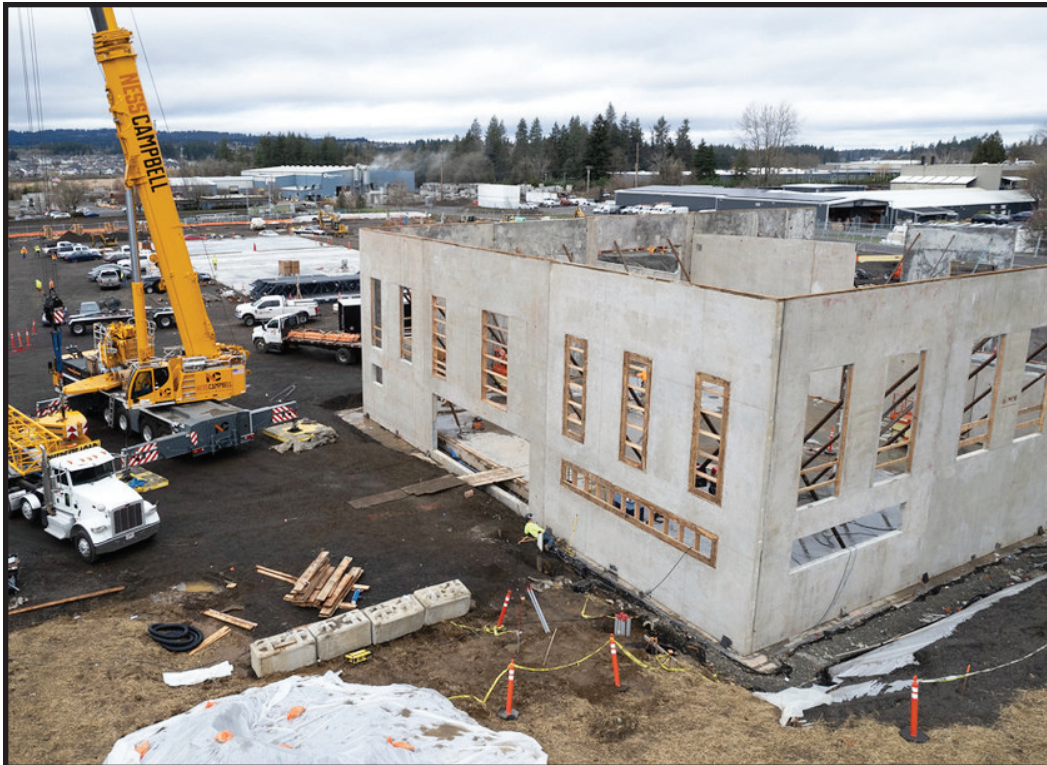
Public Works Complex: Building A with tilt-up concrete walls (CIP #8113). Photo Credit: Gregg Kerber.
