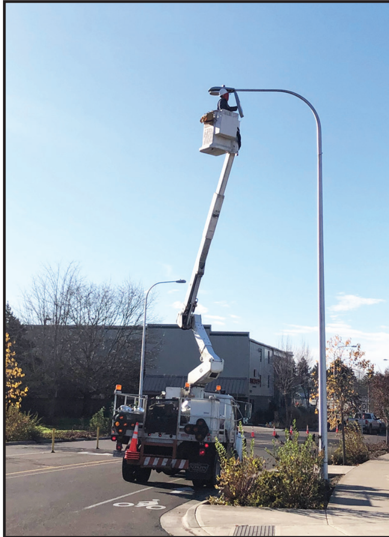
Converting from High Pressure Sodium to Light Emitting Diodes (LED) streetlights (CIP #4722).
