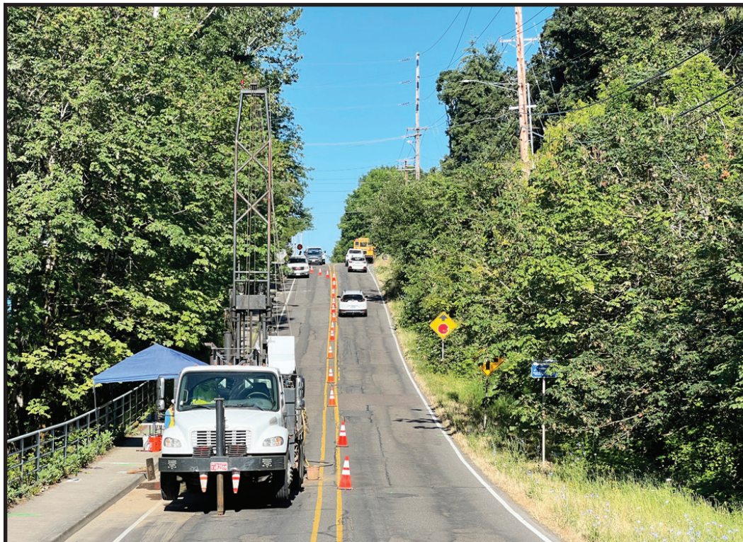
Geotechnical boring in the Boeckman “dip” where bridge piles will be installed (CIP #4212).
