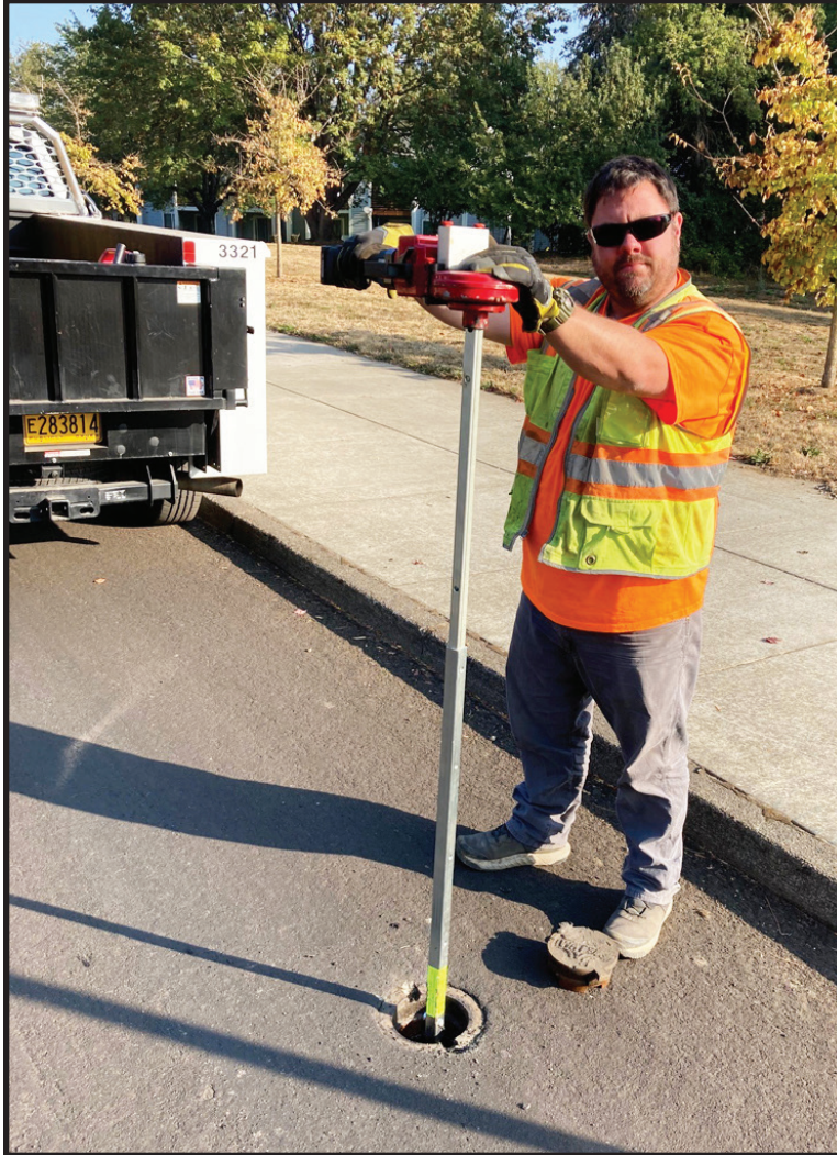
Water Distribution Technician Chad Whiting exercises a mainline water valve.
