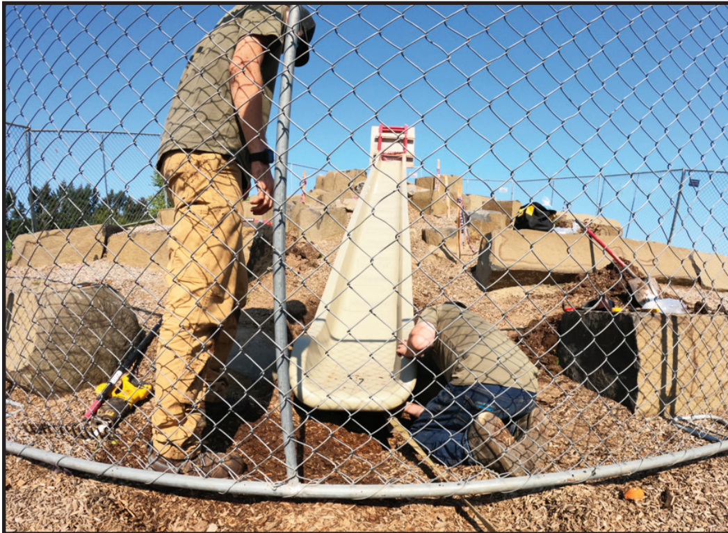
Parks team repairing the slide at Murase Plaza to ensure a safe and well maintained playground for the community (CIP #9152).
