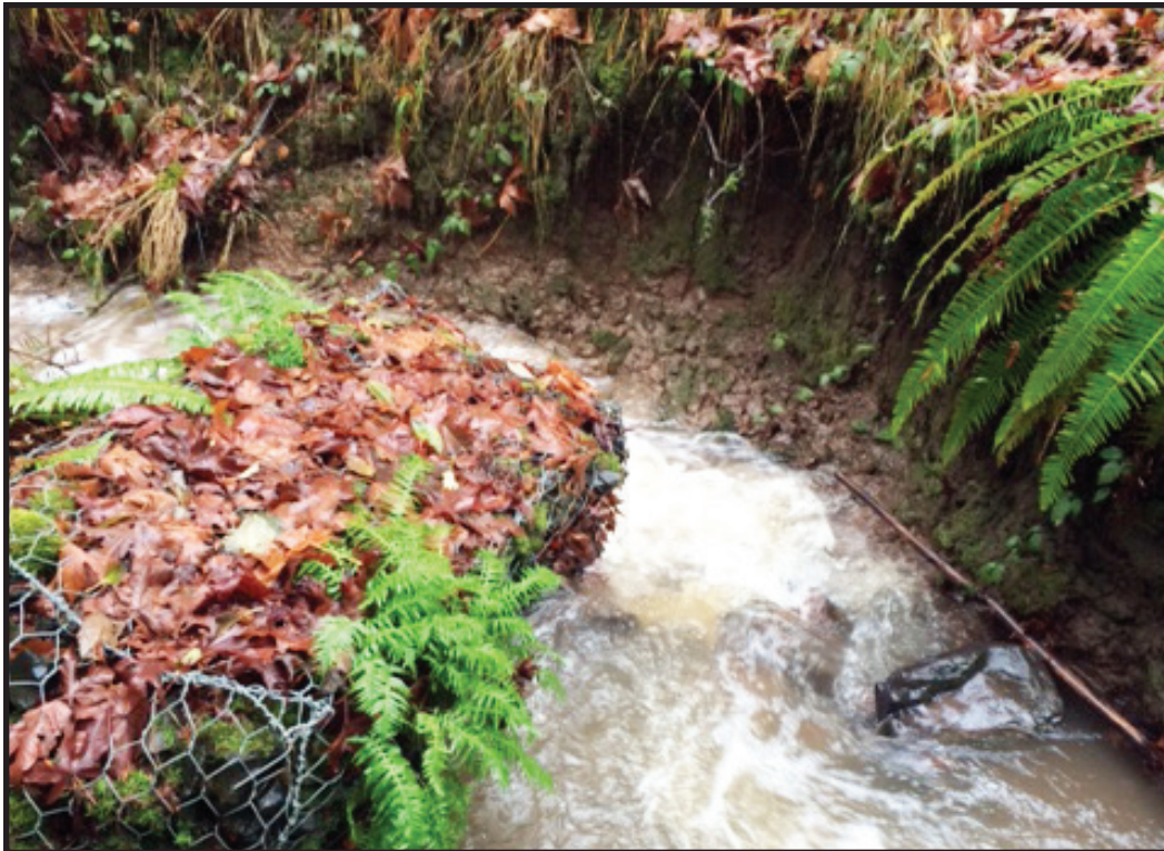
Active channel erosion undermined previous streambank stabilization measures (CIP #7054).
